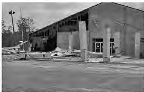
Exterior Damage - Habibi Temple
