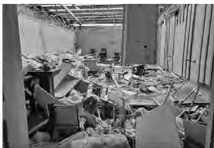
Interior Damage - Habibi Temple
